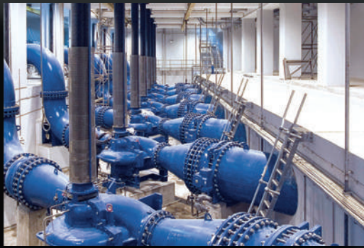
Pumps and compressors
